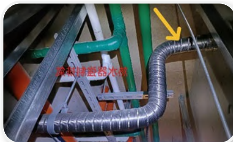
Forced Exhaust System for Water Heaters
