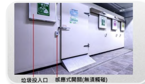
Garbage disposal chute
