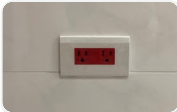
Emergency Power Outlets
