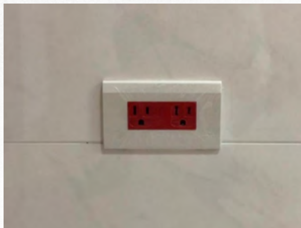
Emergency Power Outlets
