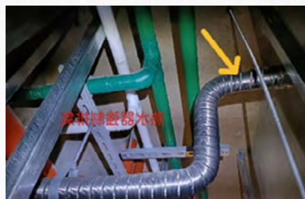
Forced Exhaust System for Water Heaters
